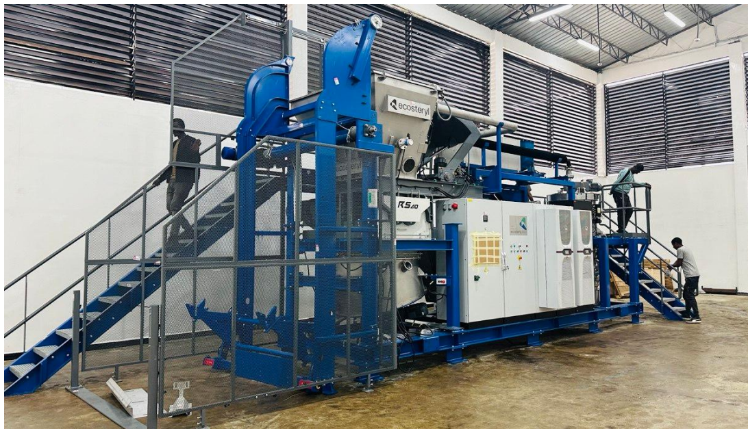
Figure 4: Current installation status Ecosteryl 250 at St. Paul Hospital and its specifications
